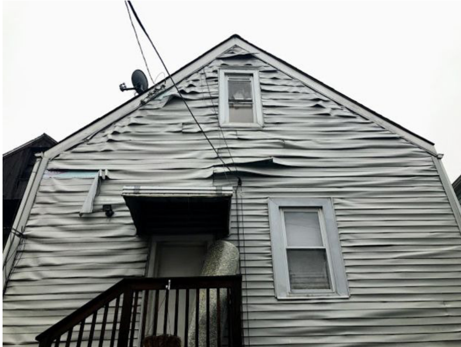
The melted siding
