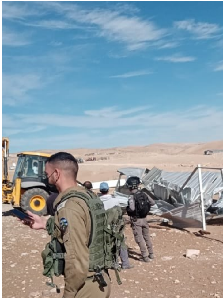
Demolition attack in Al-Fakheet, SHH
